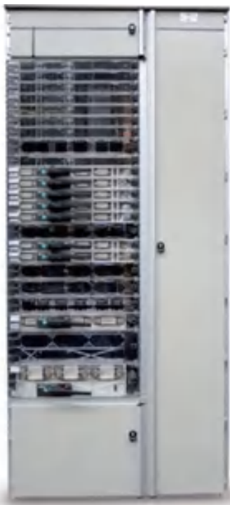
SD cabinet with fuse unit
