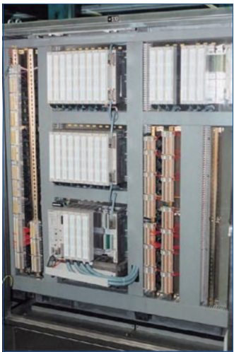
SD cabinet with fuse unit
