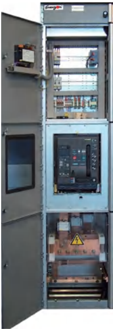
PD cabinets wt withdrawable trame drcut breakers
