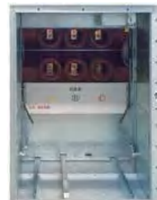
Circuit Breaker Truck Compartment
