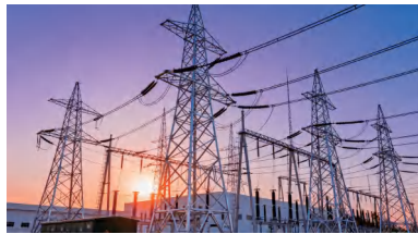
电网和配电 Power Grid and Power Distribution
