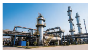
化工和石化行业 Chemical&Petrochemical Industry
