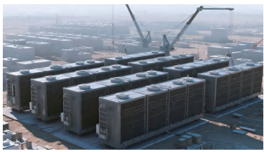
储能行业 Energy Storage Industry
