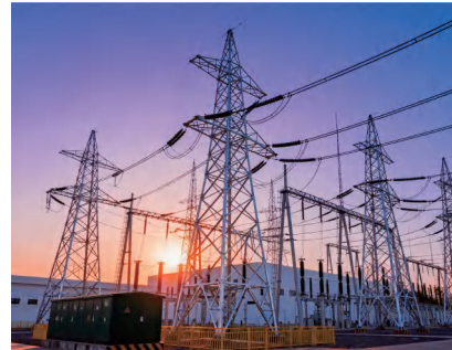
Power Grid Distribution
